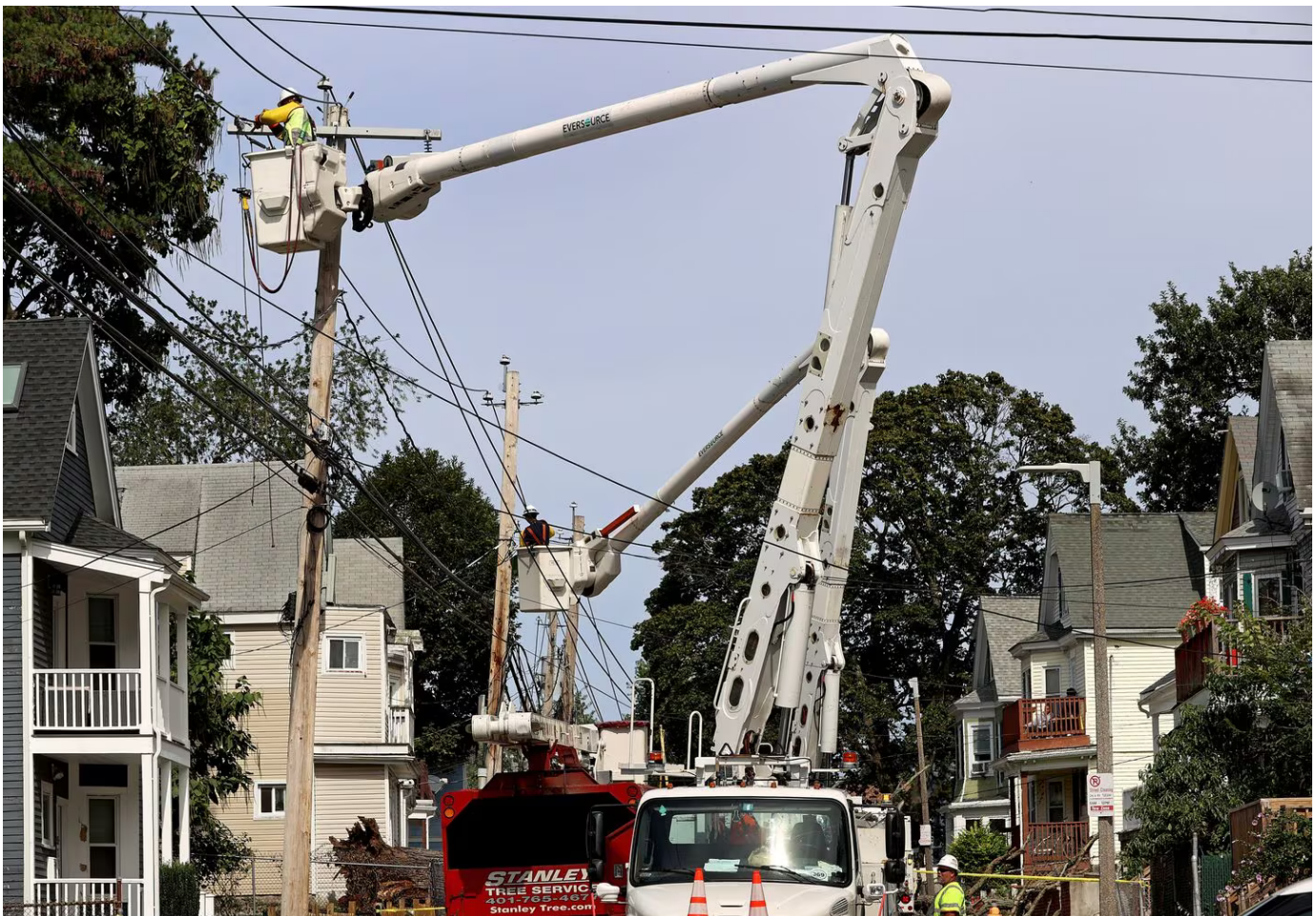
Workers repair electrical lines affected by a fallen tree in Dorchester on Sept. 15, 2023. Forty percent of residents in
